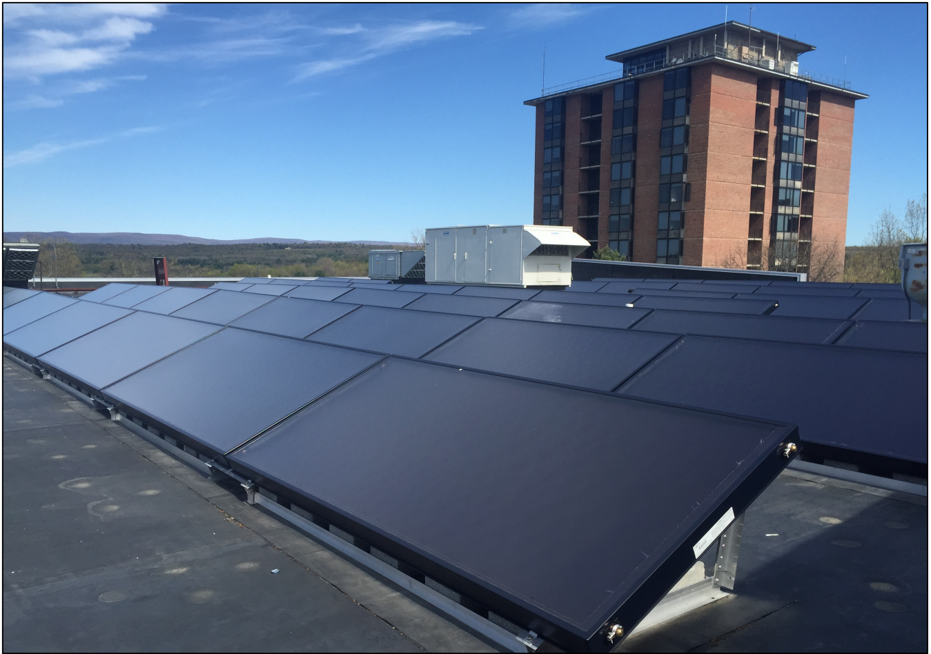
Skidmore's 54-panel solar thermal array
