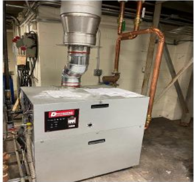
New Domestic hot water boiler installed
