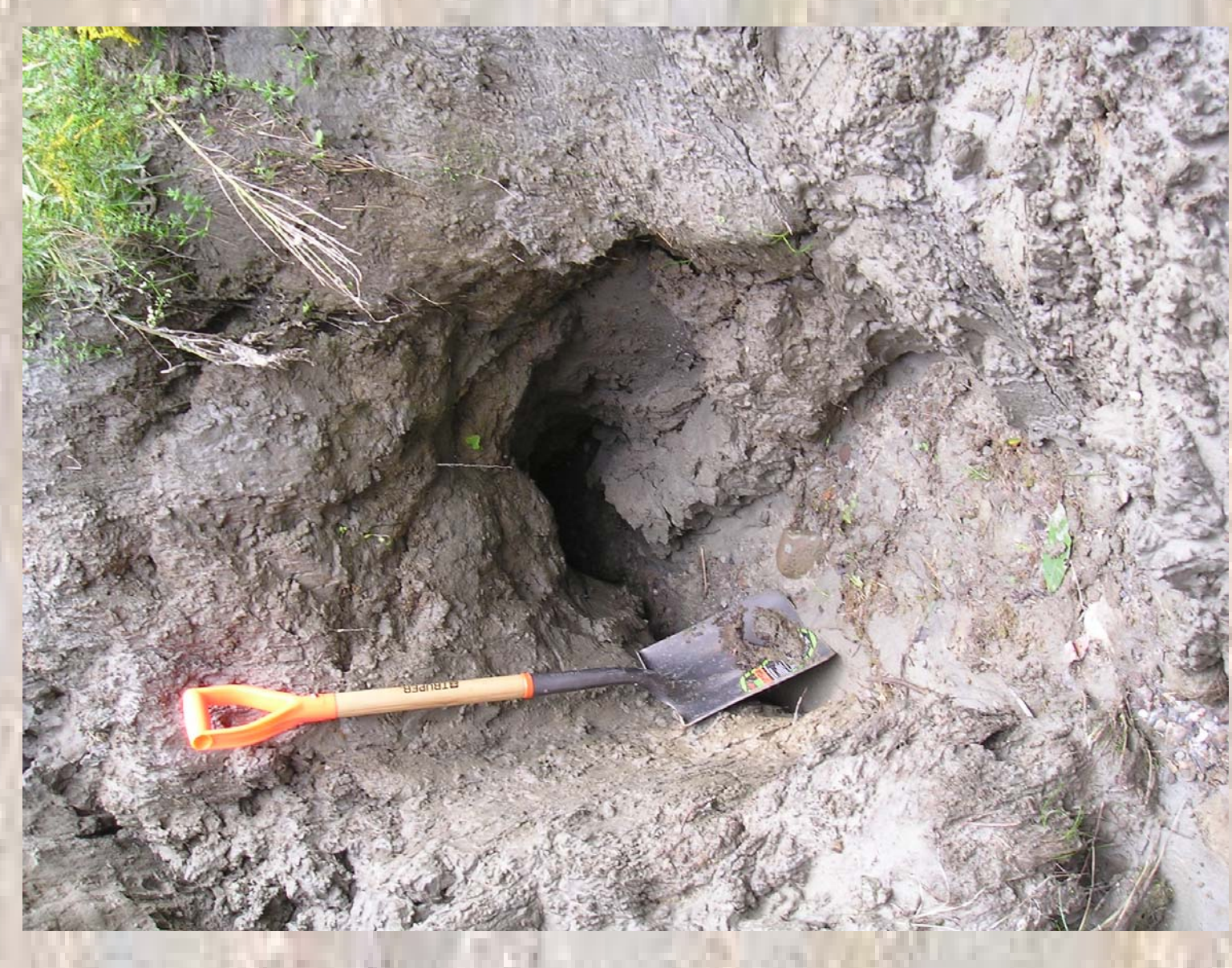
Collapsed pipe at bottom of gully
